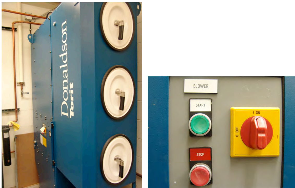
Figure 4. The dust collector and its control panel in Room 17C.
