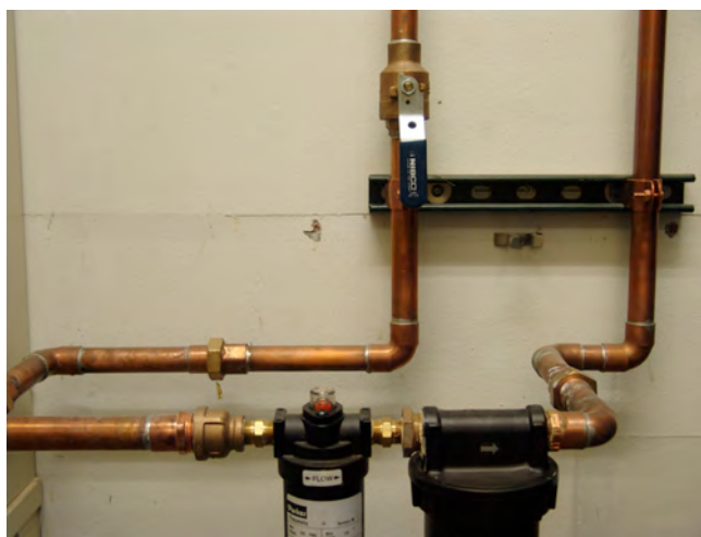
Figure 3. The main compressed air valve in Room 17C. Note that the air is turned on.
