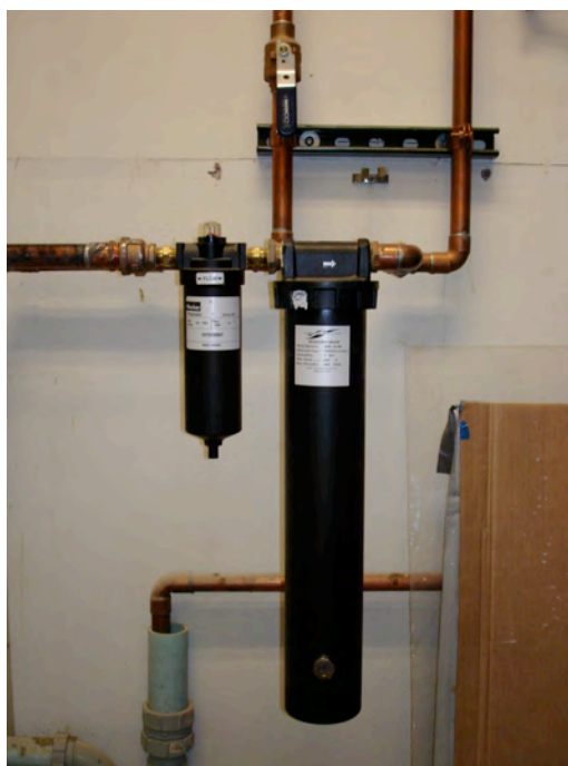
Figure 11. Air filter and air dryer
